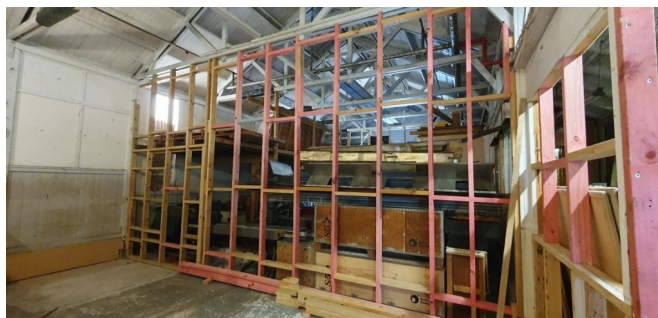
This photo shows the final wall fully framed up. All the timber in this wall is fully borer treated (H1.2)
