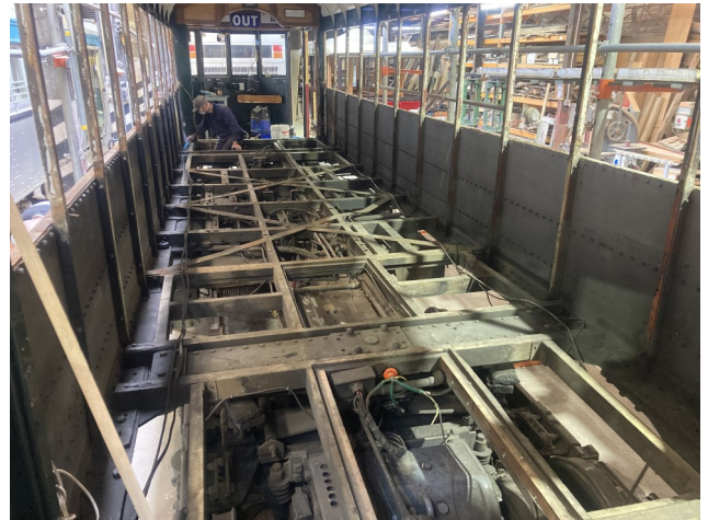
The interior during the stripdown, Woodworker Leighton removing the last of the flooring.
